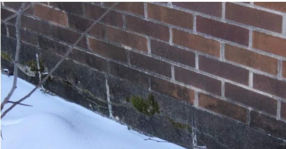
Photo #6: Enlarged view of damaged CMU at base of building.
