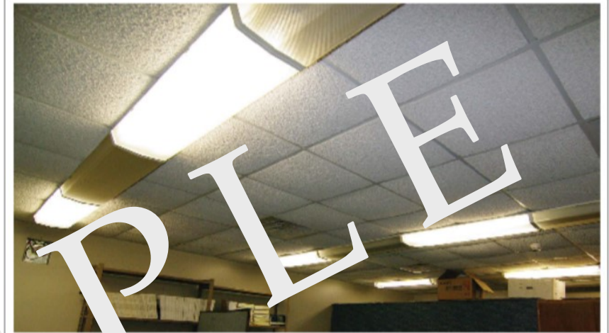
sagging ceiling tile
