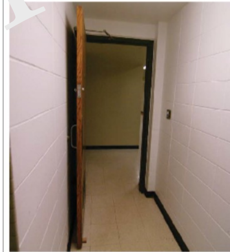
non-ADA compliant door at restrooms
